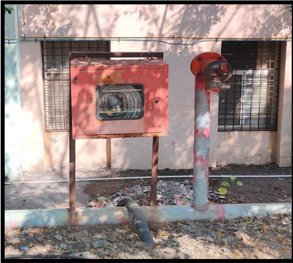
FIRE FIGHTING SYSTEM
